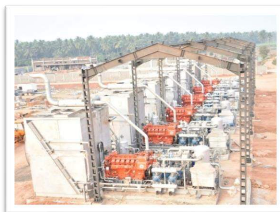
Gas Compression Station, GITL Tadepalligudem
