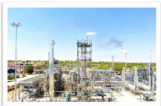
RGT Bridge Plant Cairn Vedanta Barmer, Rajasthan
