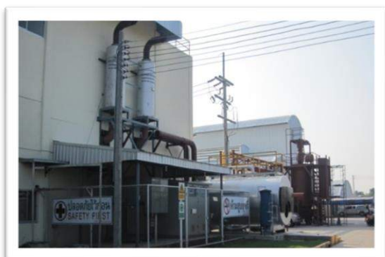
Biomass Power Plant- Satake International, Thailand
